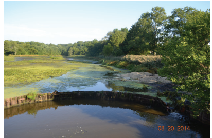
A notch cut in the dam (seen far right) allowed the water to slowly decant while retaining sediments in the pond. This project is now close to completion.
